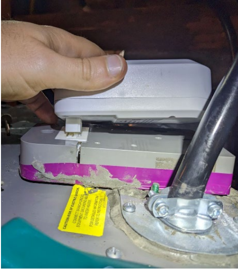
Figure 1. UCM being plugged into a 240V HPWH.
